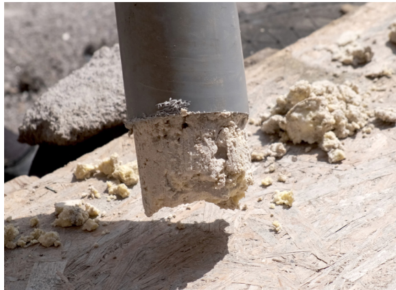
Pipe clogged with fats, oil and grease
