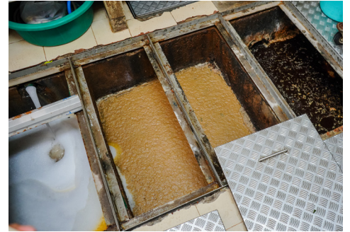
Commercial Kitchen Grease Interceptor
